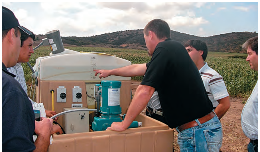
TRAINING. A chemigation system featuring a Neptune Series 500 metering pump is perfect for use with a center-pivot watering system due to the pump's ability to deliver precise amounts of fertilizers and chemicals at the precise time.
